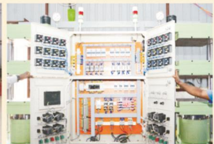
ELECTRICAL PANEL BOX
